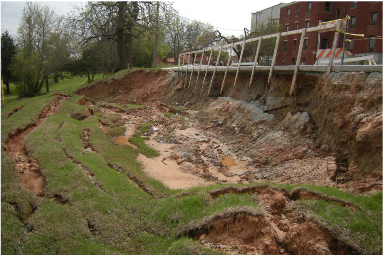
Photograph #3: ECU Slope Failure
