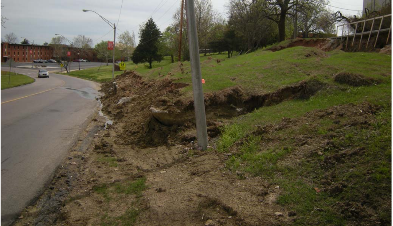
Photograph #2: ECU Slope Failure
