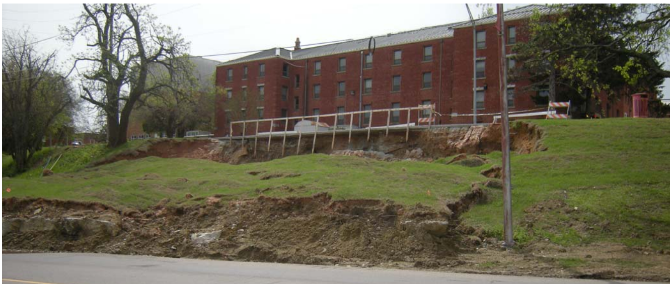
Photograph #1: ECU Slope Failure
